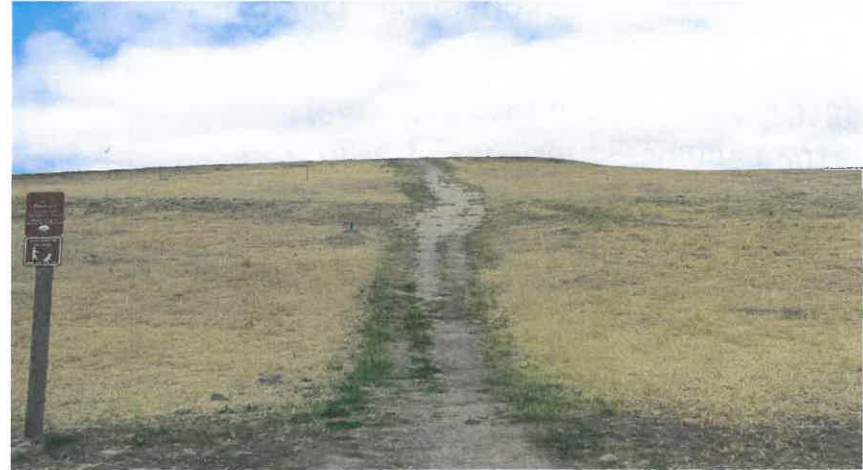
Progression of erosion caused by unauthorized uses on landfill cover
